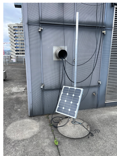
(b) Outside: Solar panel.
